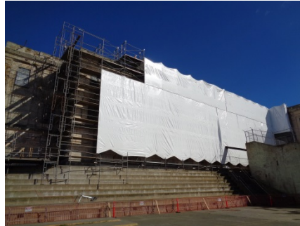
Shrink wrapping provides a visual barrier so that work does not disturb the island's birds.
